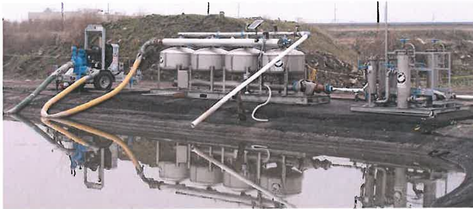
Figure 5. Sand filters (center) and bag filters (right) prior to discharge to waterway.
