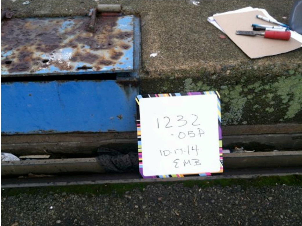
Photograph 7: Pier 4, Bullrail Box - Blue (Sample 1232-05P)
