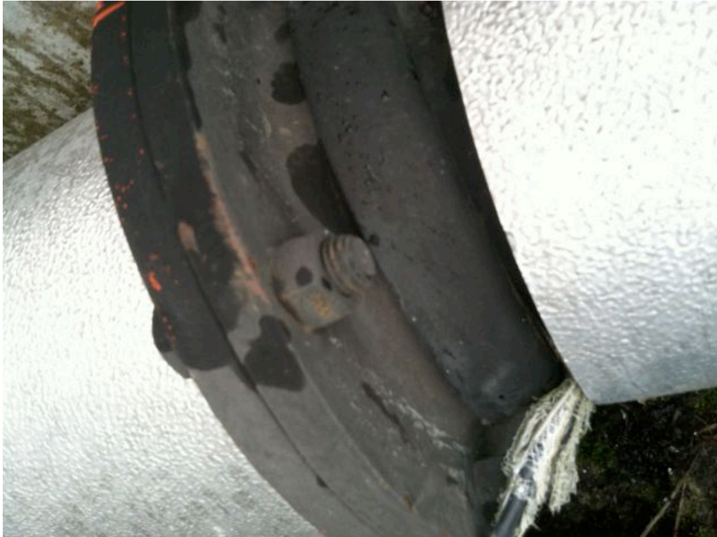
Photograph 1: Pier 4, Wire Wrap inside Ducted Pipe (Sample 1232-01A)
