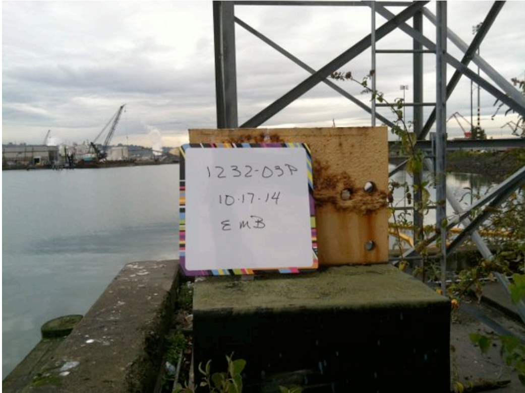
Photograph 5: Pier 4, Anchor Box - Yellow (Sample 1232-03P)
