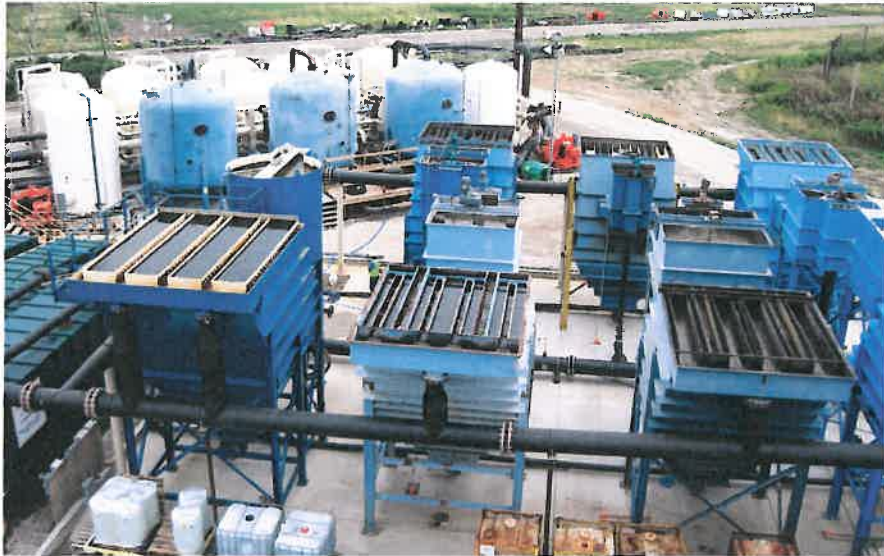
Figure 8. Aerial view of the WTP equipment during operations.
