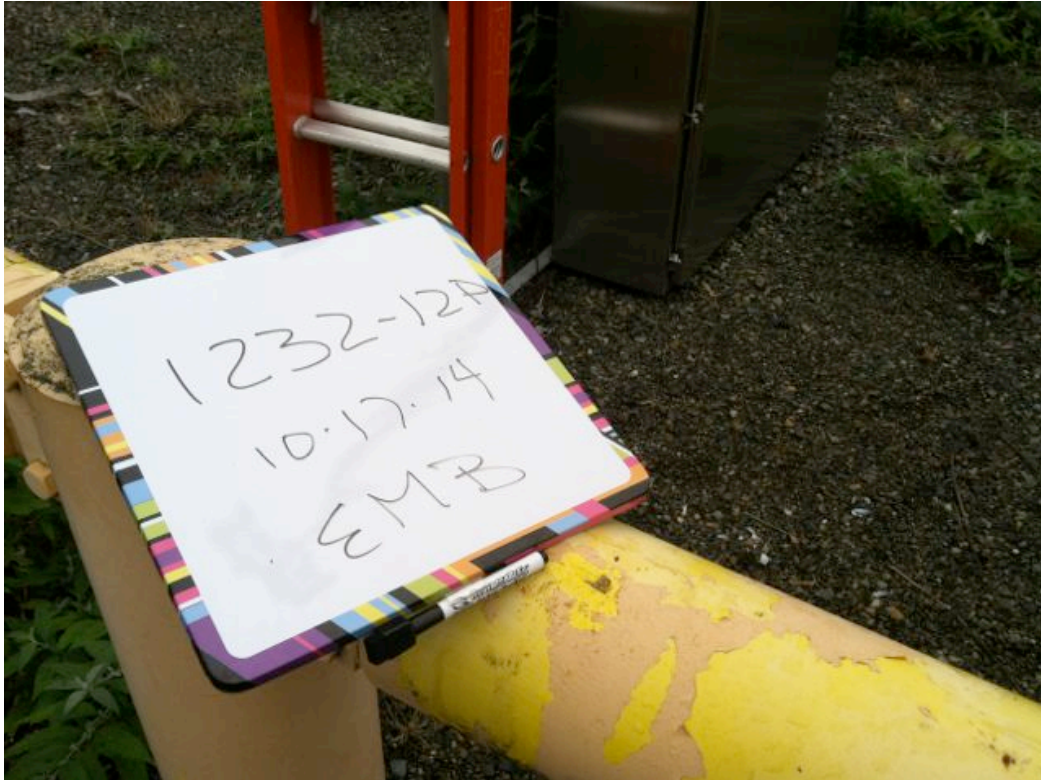
Photograph 12: Pier 4, Railing at Substation –Yellow (Sample 1232-12P)
