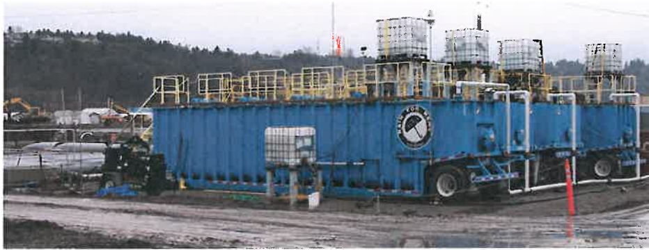
Figure 3. Mixing tanks, upland sediment capture system.
