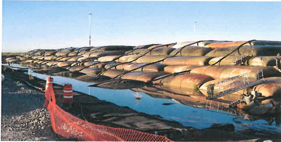
Figure 5. Non-TSCA dewatering pad with geotextile tubes stacked in 5 layers.
